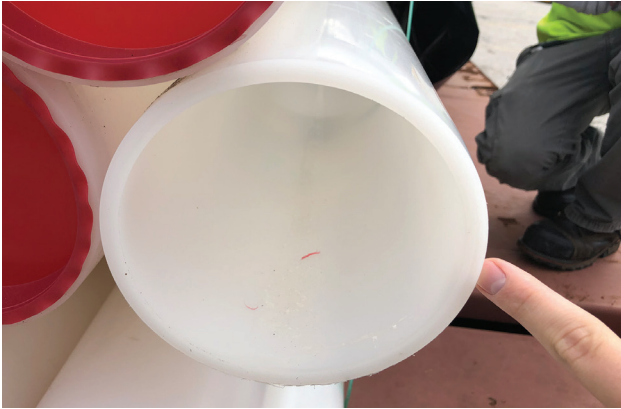
↑ Figure 6: New Kynar PVDF pipe replaced 316 stainless steel. 📷 Courtesy of Simtech Process Systems
