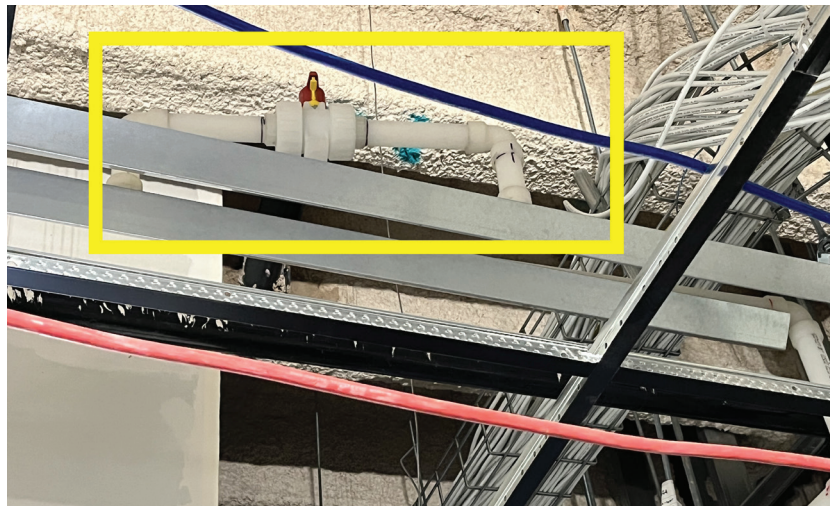
PVDF system (highlighted in yellow box) installed in plenum. Photo courtesy of MTech Mechanical
